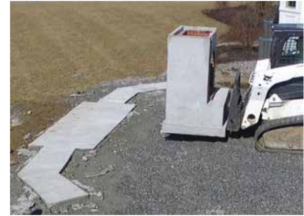
Step 3: Place units on footings. Use refractory cement to adhere cap to base.
