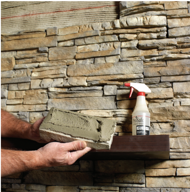
Top: Grid the wall with chalk lines. Above: Apply mortar to back of stone. Above right: Keeping the stone level, wiggle into place.
